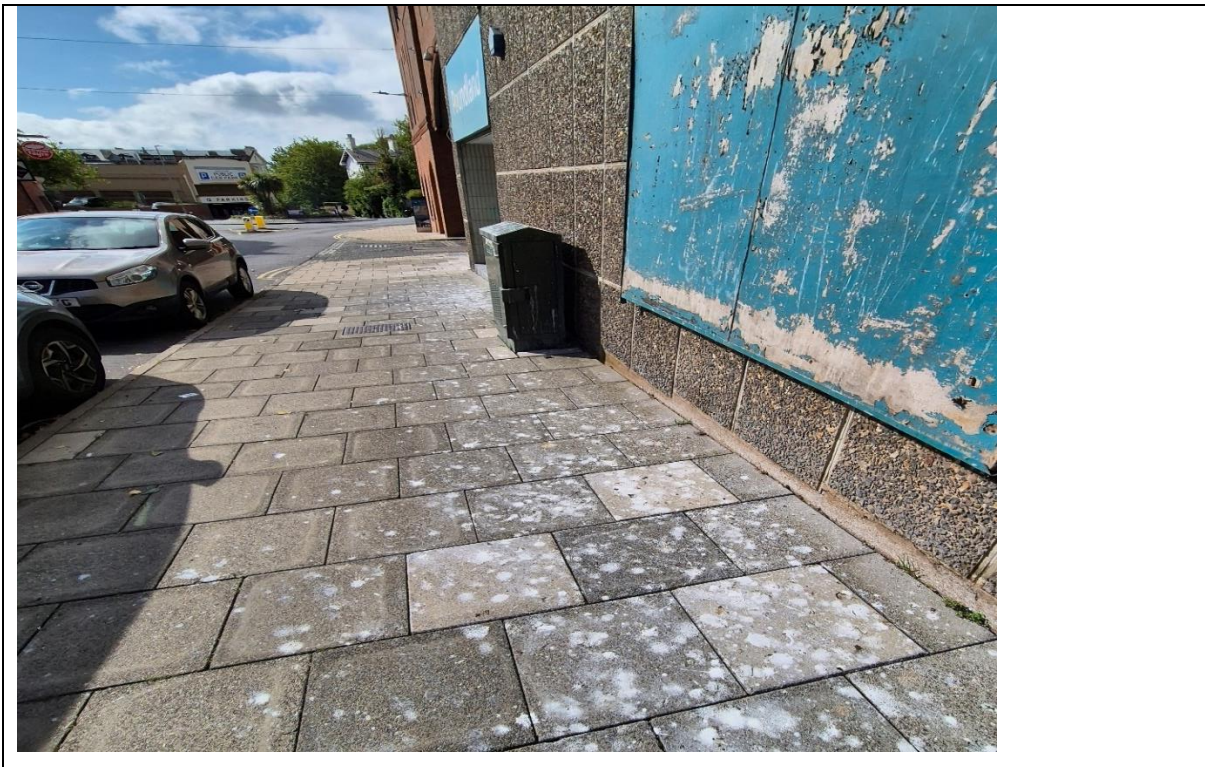
Figure 14: A 'hot spot' area of pavement prior to jetting in Scarborough town 2025.
